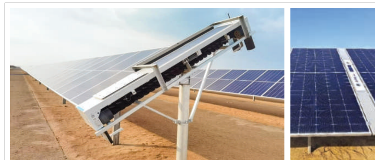
Figure (2): Robots Working on the Modules While the DustIQ Examines their Efficiency – Source: Sunpure
