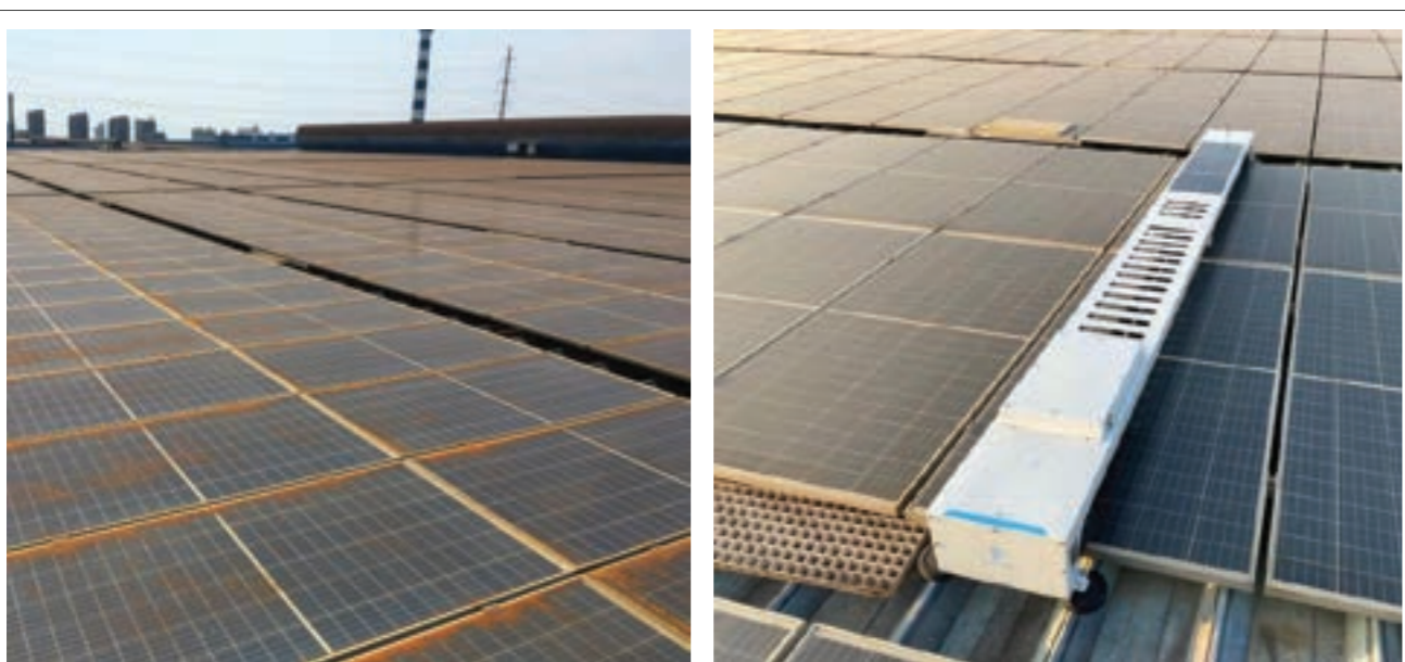
Figure (1): The Modules on the Rooftop PV Plant were Covered with Metallic Dust, Leading to Rusting. Regular Cleaning by Robots Significantly Improved the Situation of the Modules – Source: Sunpure
